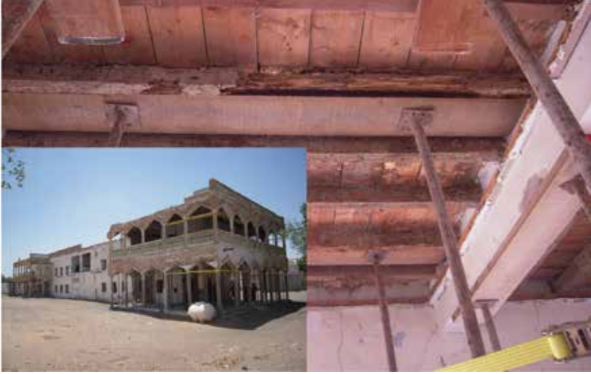
Heritage building has its wooden structure weakened by termites (Image courtesy of José Luiz Pedersoli Jr.).
