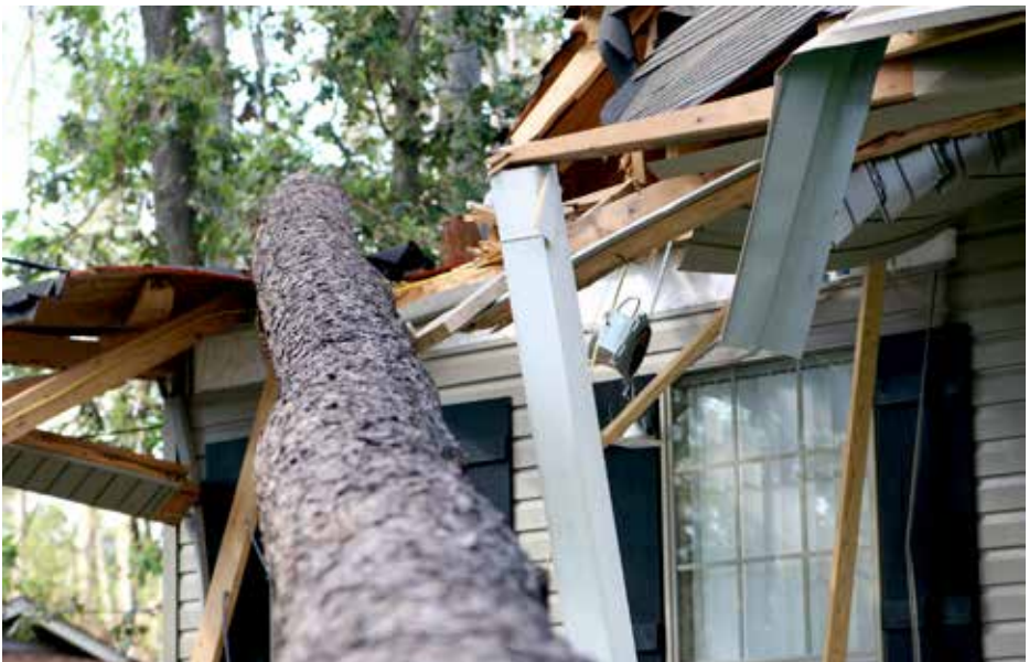
Examples of dangers to heritage assets at the different layers of enclosure. Large trees around a heritage building can fall on it causing serious damage (site) (istock.com/barmixmaster).
