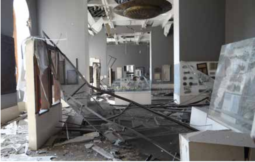
Extensive damage to a museum collection caused by a bomb blast (Image courtesy of AbdelHamid Salah, EHRF - Egypt).
